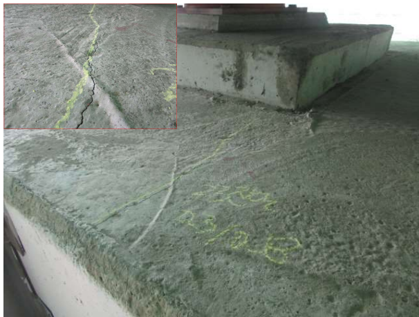
P7 균열( Cw=0.3/L=0.8m )
