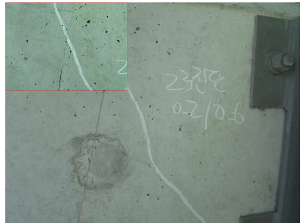
P1 균열( Cw=0.2/L=0.6m )
